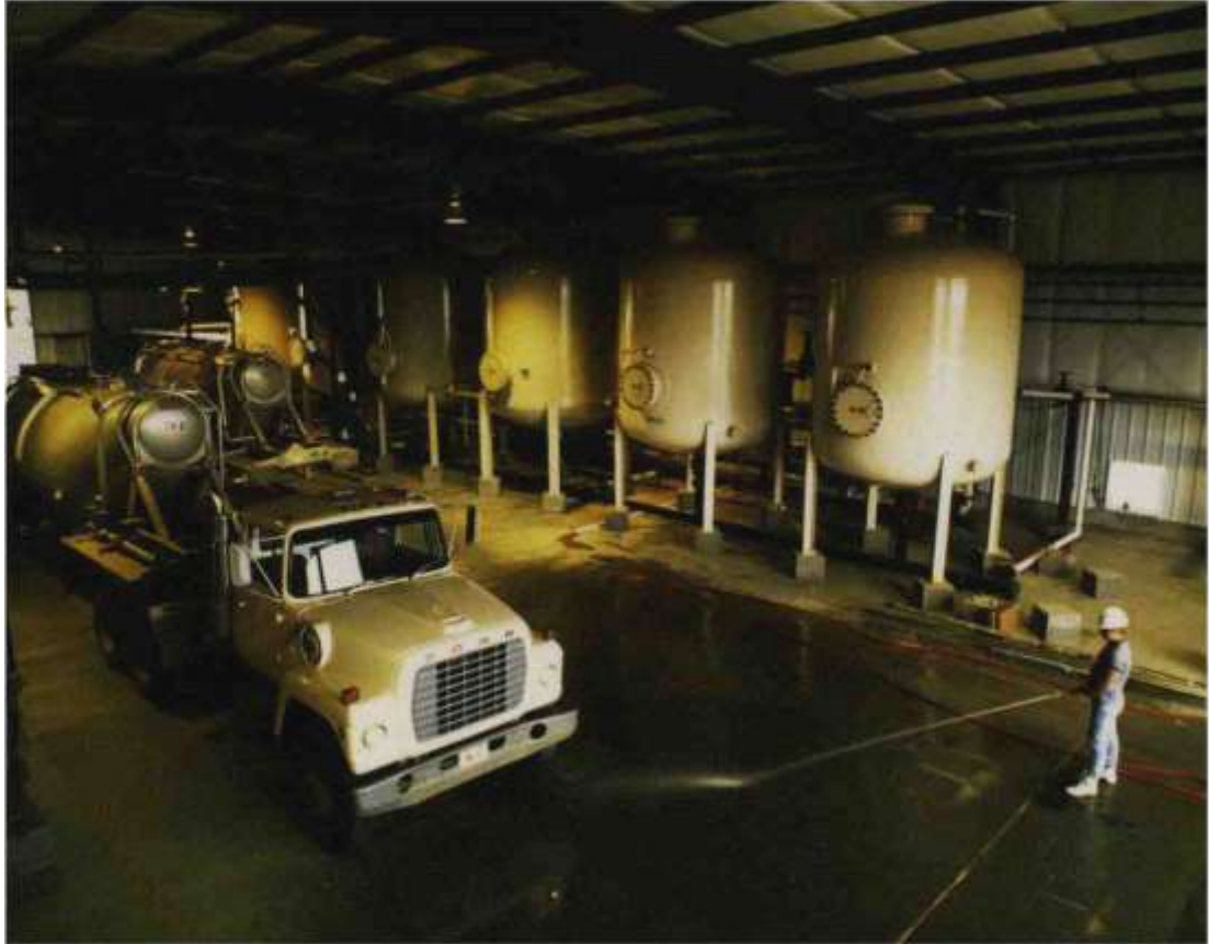
Figure 15 Satellite Ion Exchange Columns with Resin Trailer –
