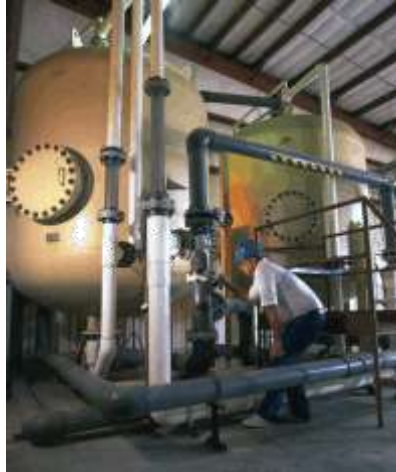
Figure 11 Ion Exchange Columns –
